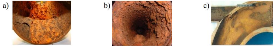
Fig. 1 Internal corrosion: a) localized pits 1 , b) fouling 2 and c) wear/erosion 3
