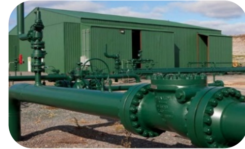
Compressor and Pump Stations
