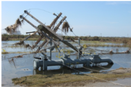
Pipeline manifold impacted by flooding
