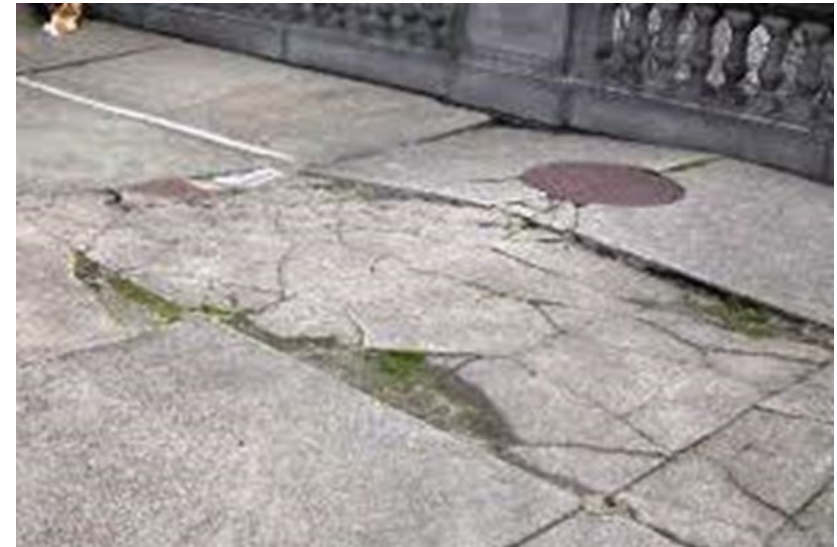
Frost Heave at Pavement Surface
