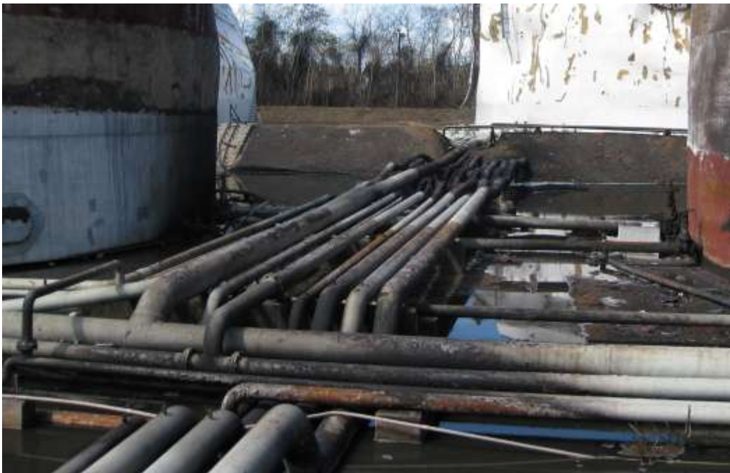
Figure 145: Close up of pipework in the area in which transition occurred
