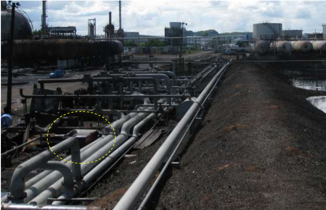
Figure 107: Depressed steel cover indicating moderate to high overpressures (marked as No. 1 in Figure 106)
