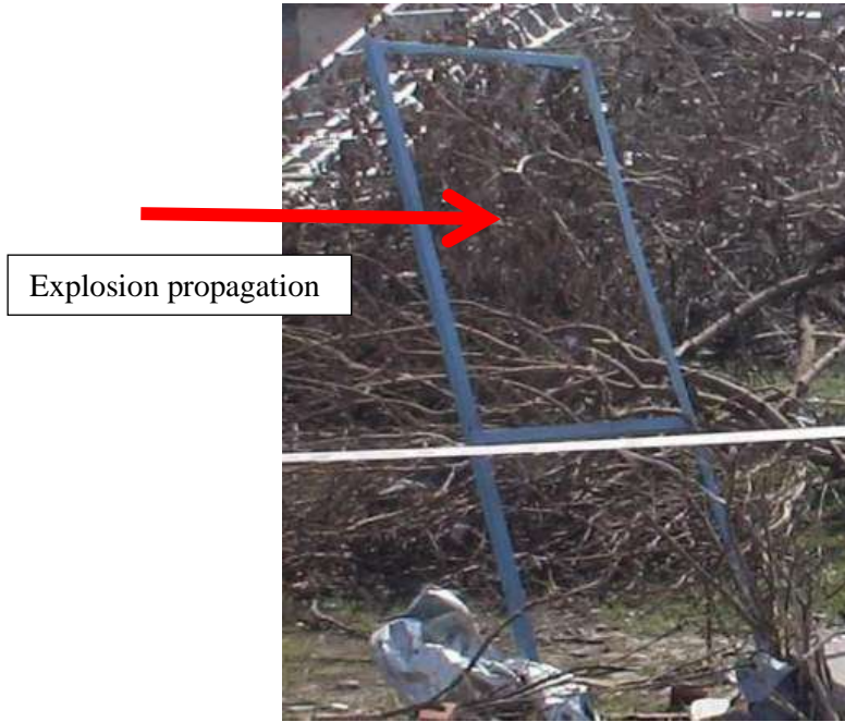
Figure 234: Backwards deflection of a steel support frame at Jaipur
