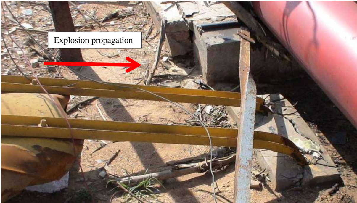
Figure 236: Backwards deflection of a steel support frame at Jaipur
