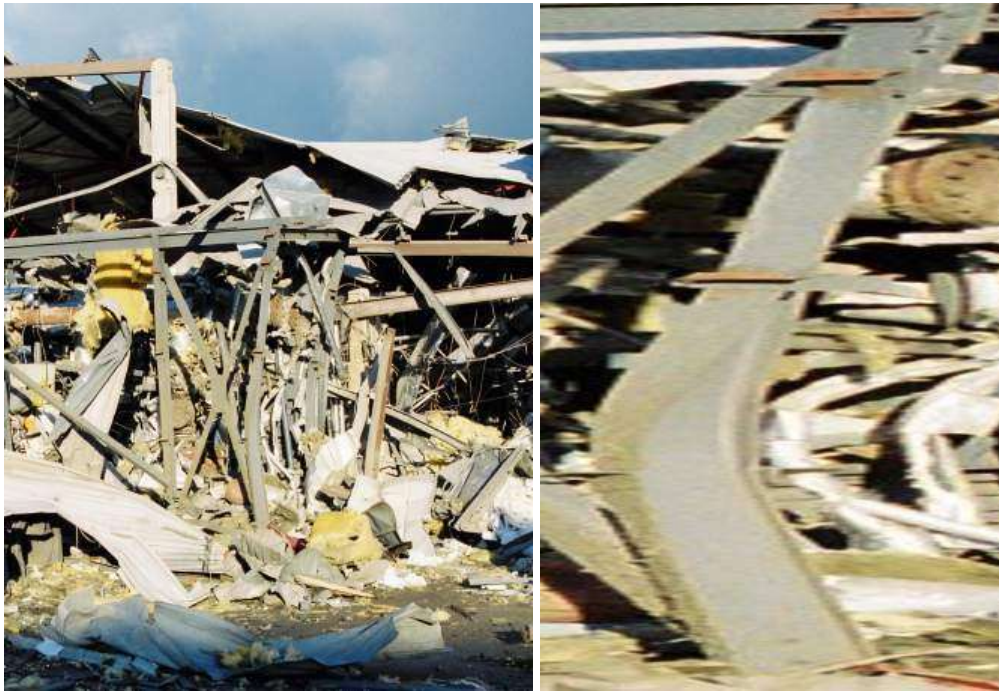
Figure 82: Deformed steels outside and within the Buncefield cloud exhibit hinged failure – characteristic of loads applied over a long period relative to the natural frequency
