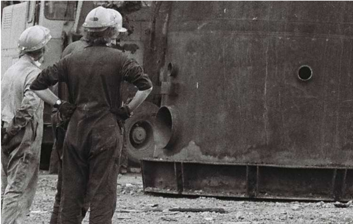
Figure 68: Reactor 2. Limited pressure damage to reactor skirt
