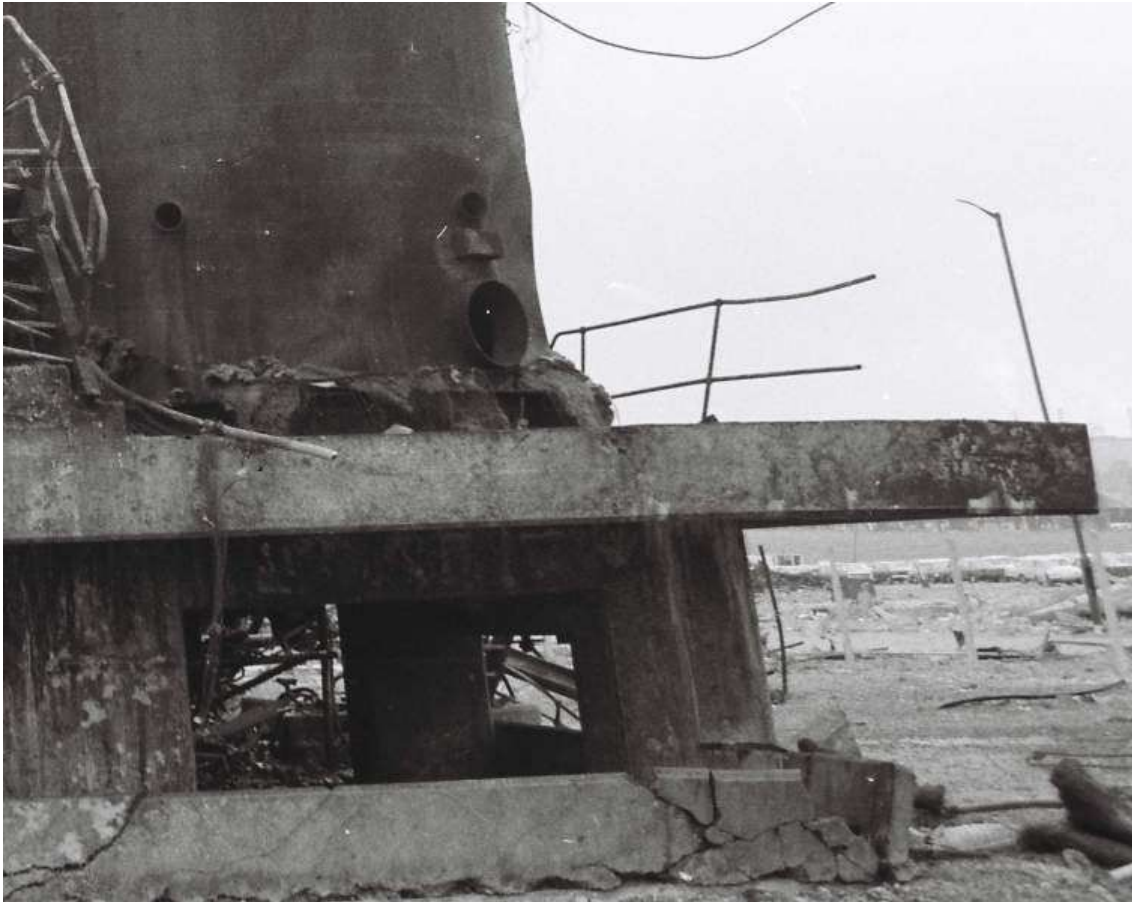
Figure 70: Reactor 6 (Number 5 missing). Significant pressure damage to the skirt
