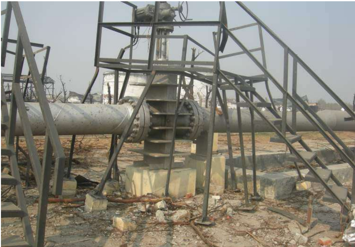
Figure 207: Lightweight open steel structures in the centre of the Jaipur explosion – there no evidence of continuously curved steels that were observed in detonation testing.
