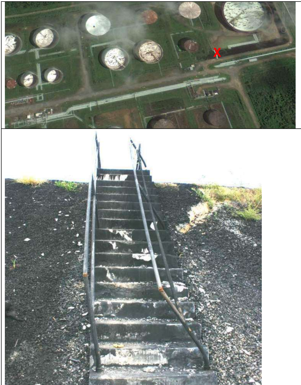
Figure 113: Deformed handrail indicating high overpressures (marked as No. 7 in Figure 106)
