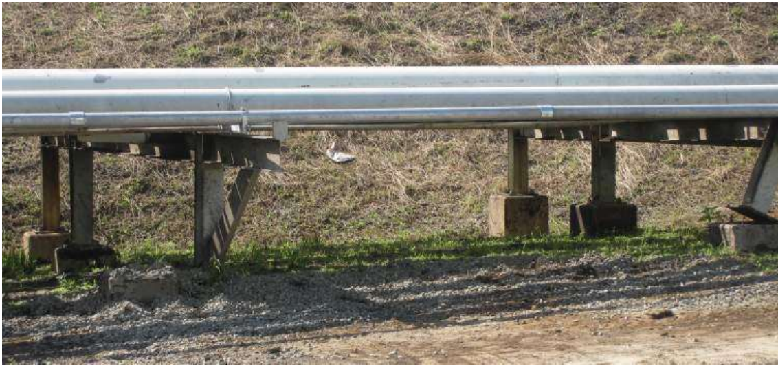
Figure 111: Displaced pipe supports indicating moderate to high overpressures (marked as No. 5 in Figure 106)
