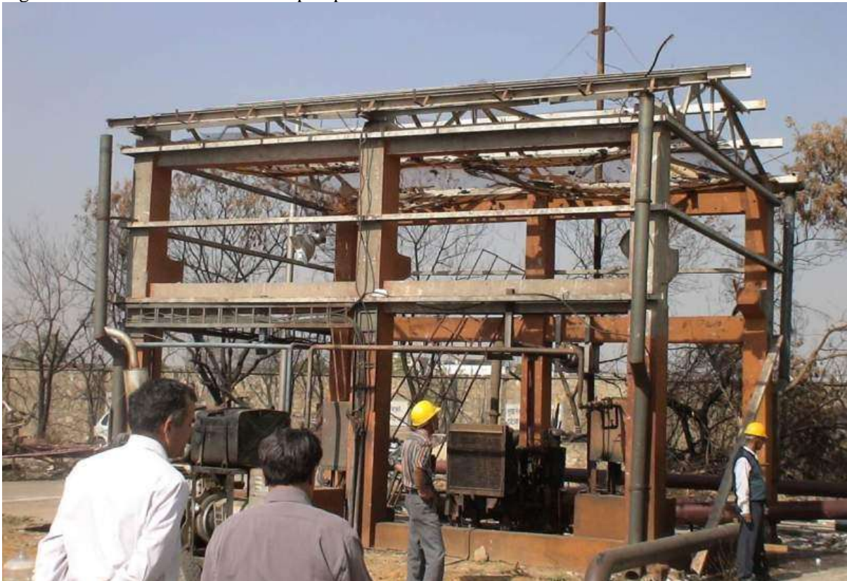
Figure 19: Remains of the pump house on the edge of area affected by the severe explosion.
