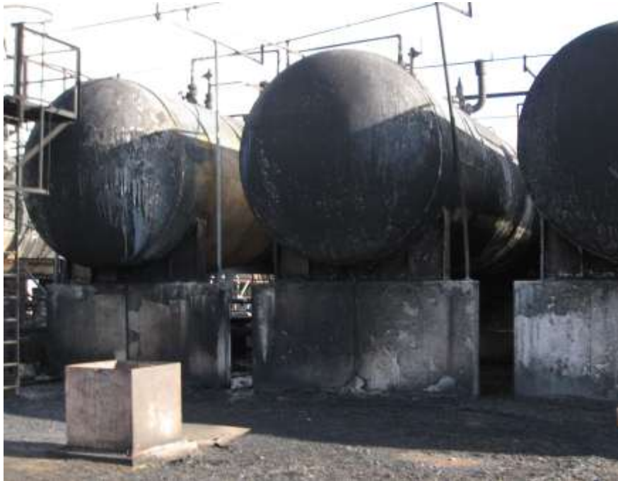
Figure 99: Low level of pressure damage to pipes and steel box
