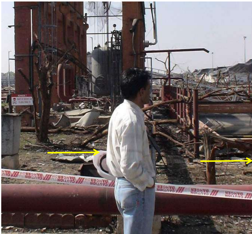
Figure 22: Broken trees near the pump house. Arrows show direction indication
