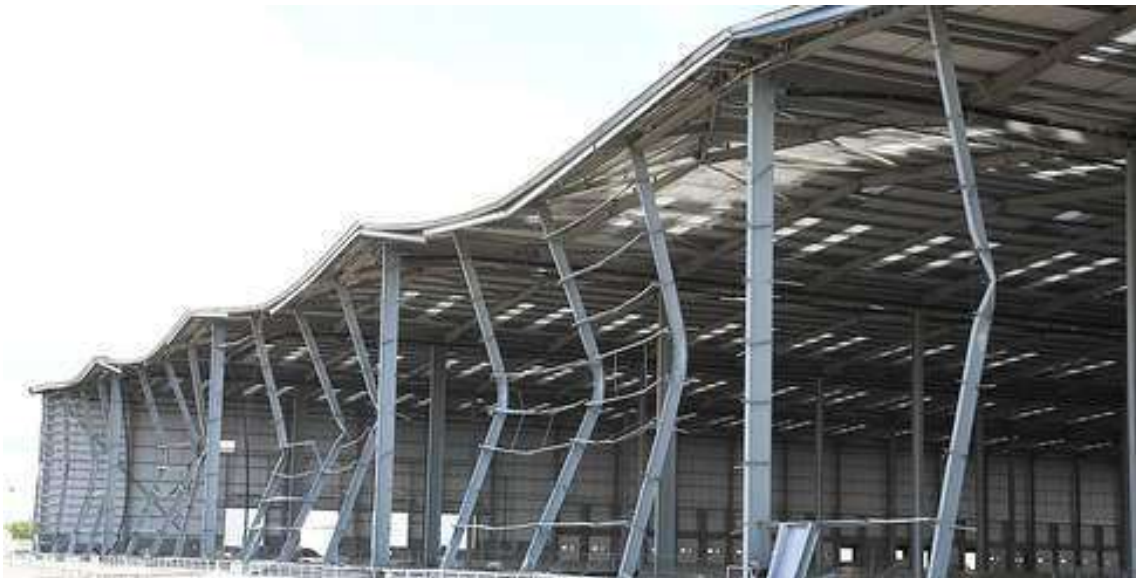
Figure 46: Deformation of the front face of a building about 300 m (984 ft) from the edge of the Buncefield cloud.
