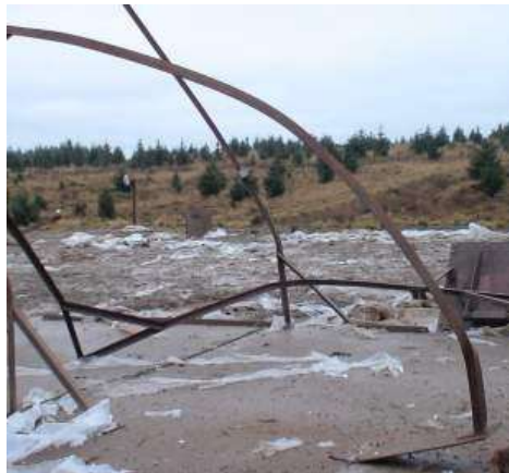
Figure 73: Angle iron deformed by a detonation (depth 3m)
