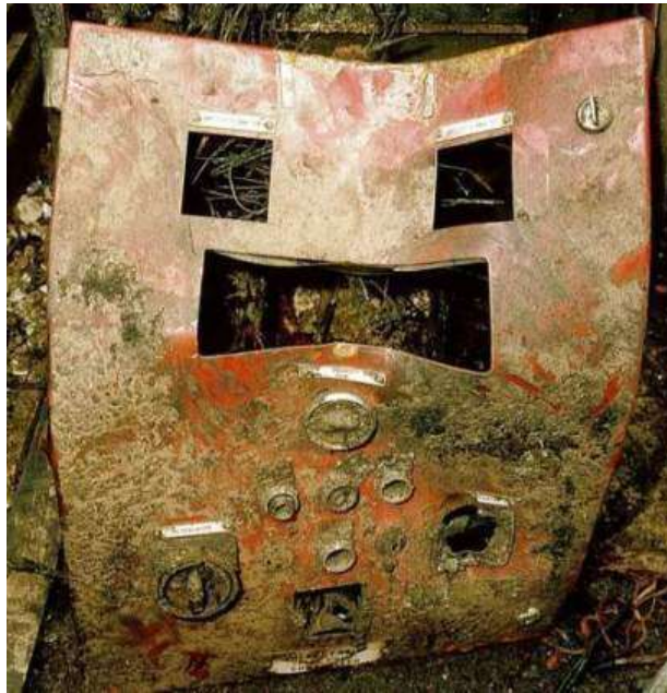
Figure 32: Pressure damage to the front of the enclosure of the diesel pump starter
