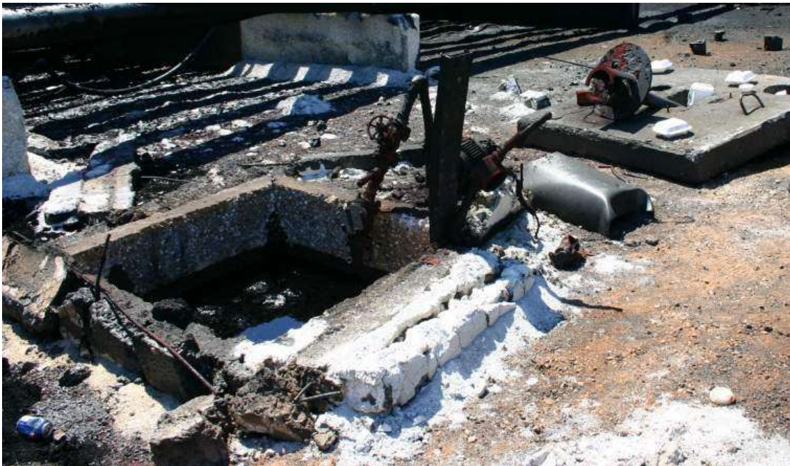
Figure 105: Displaced drain slab at the East end of “D” Street.
