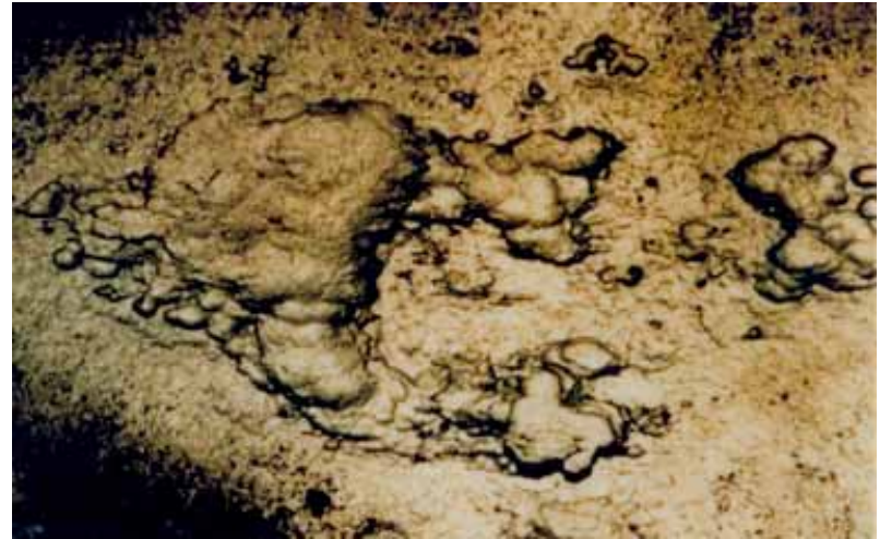
Close-up of sand-blasted surface showing MIC pattern
