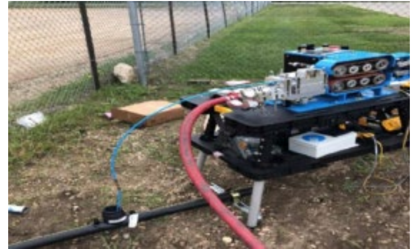
Prototype Testing of Pneumatically Driven Duct Rod Pusher Propelling Duct Rod into a Pipeline. Picture courtesy: Gas Technology Institute.
