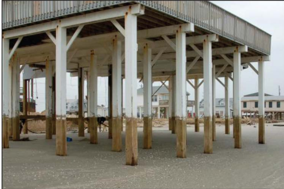
Erosion beneath elevated coastal structure from single storm event (Hurricane Ike, Galveston, TX; 2008).
