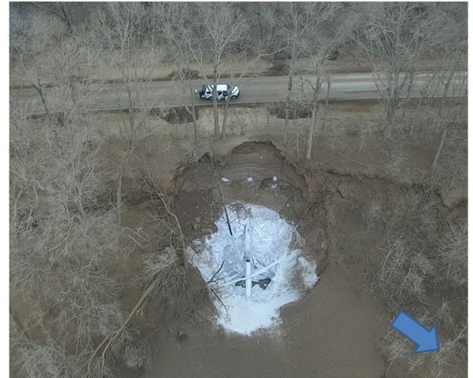
Figure 2: Vehicle is Parked on HWY 433 - The White is Ice Generated by the Release of CO 2 - The Blue Arrow Points North (Aerial Drone Photograph Courtesy of the Mississippi Emergency Management Agency)
