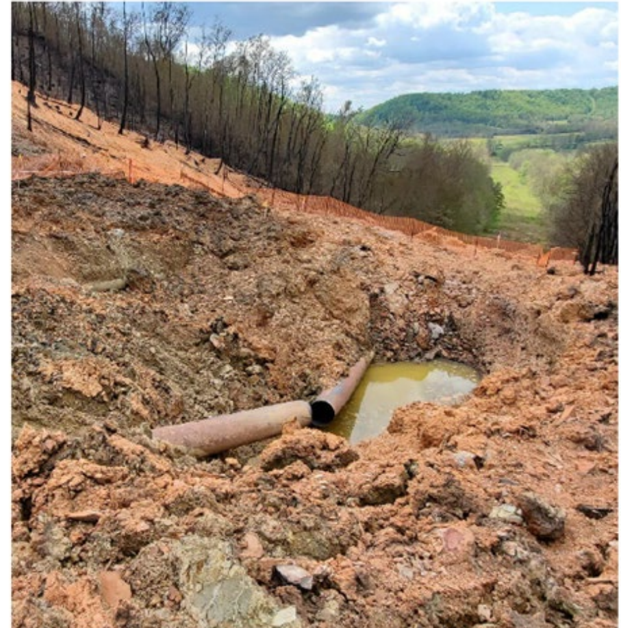
Figure 1. Ruptured pipeline. (Source: BGC Engineering USA, Inc.)
