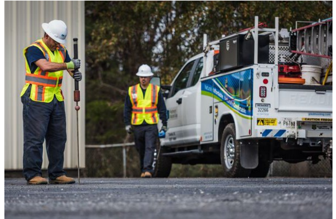
Gas technician working with gas detection equipment
