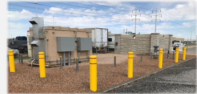
ThermH 2 – Phase 1 Facility, DEU Training Academy.
