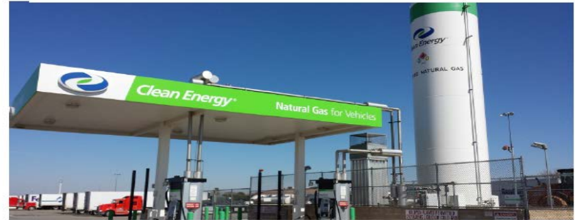
LNG Fueling Station (Source: Used with permission from Quest Consultants Inc.)
